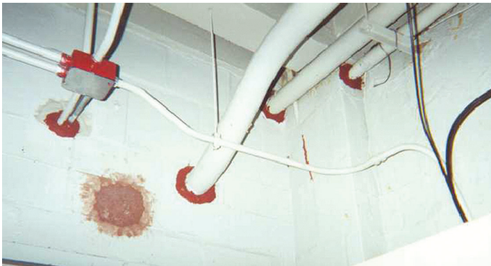
Example of proper installation of through penetration firestopping. Photo: International Firestop Council
